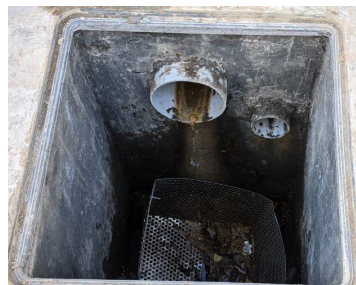
Fig. 5 Bar screen before water enters GW tank
