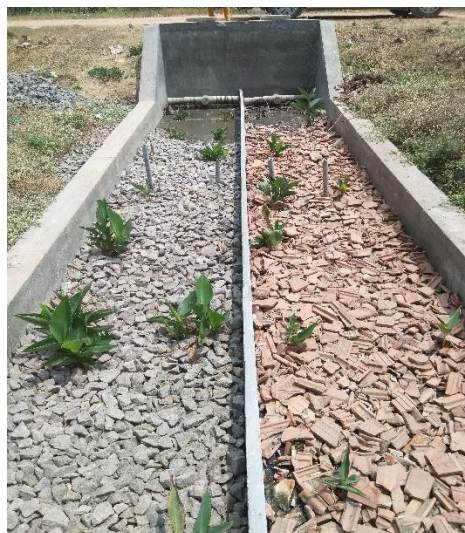
Constructed wetlands (STRAINS) to treat sewage before entering Bellandur lake, Bangalore, 2020 [Photo Credit: Ramya B]
