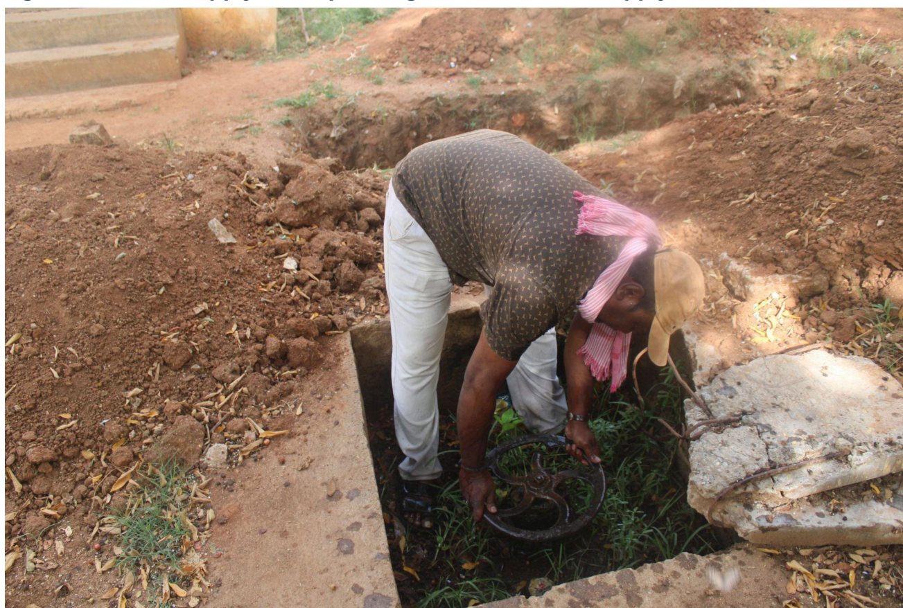
Figure 1.6: Water supply staff operating valves for water supply
