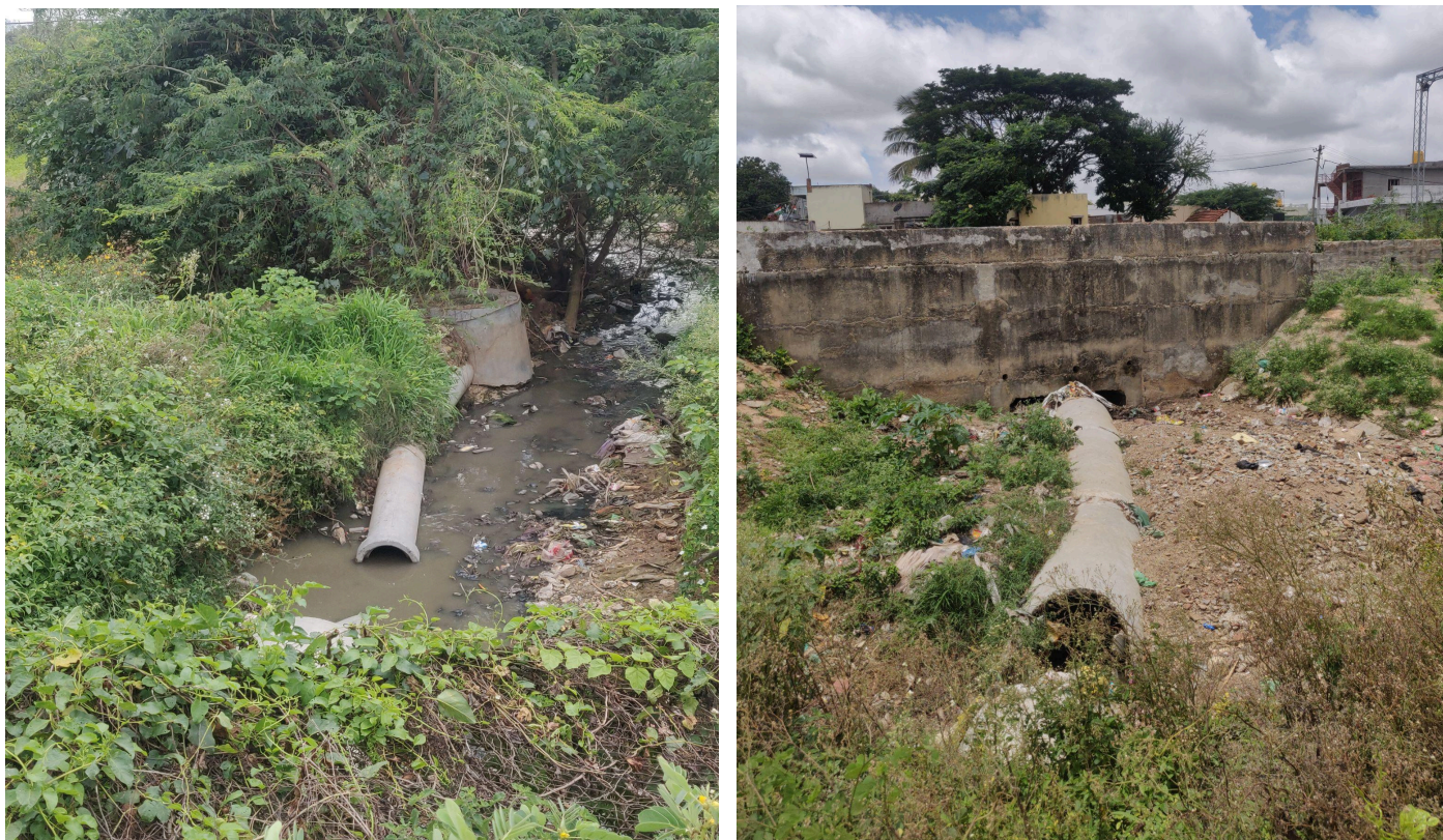
Figure 3.8 : Broken underground drainage pipes near Nekkundi lake
