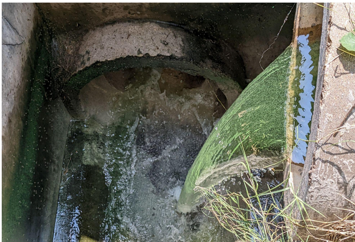
Figure 3.10: Treated water from the STP
