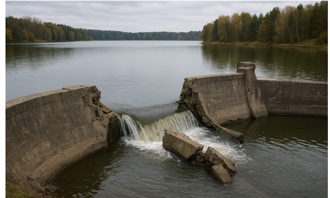
1.20. Damaged waste weir
