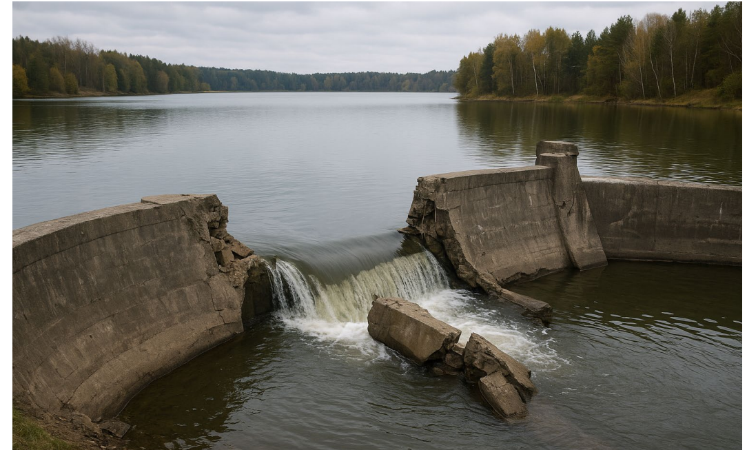
1.20. Damaged waste weir
